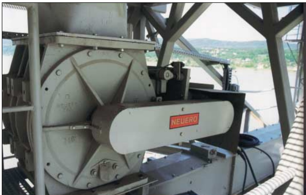
Figure 9 The blowers are driven by 55 kW electric motors
